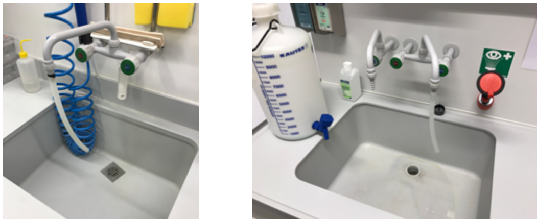
Fig. 4-2: Utility sink in use
